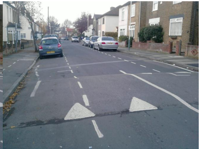
Globe Road looking towards Brentwood Road from the location of the proposed pinch poi
